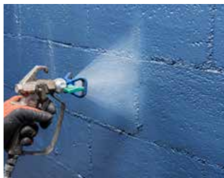
... unplastered walls, and
