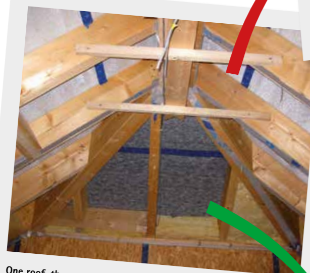
One roof, the same conditions, different results: pore-free SOLITEX MENTO membrane on the hip roof, microporous membrane on the main roof surfaces to the left and right.
